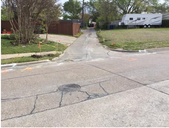
Briar Hollow / Stony Brook Alley Before Repairs
